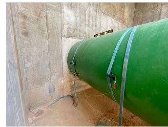
Figure 10: Flowmeter ultrasonic sensors installed in the conduct
